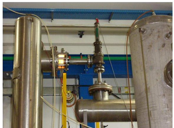
Fig. 14 – PARCOL safety relief valve during discharge test at “Fluid-dynamics of Turbomachines” Laboratories (LFM) at “Politecnico di Milano” University (water test bench)
